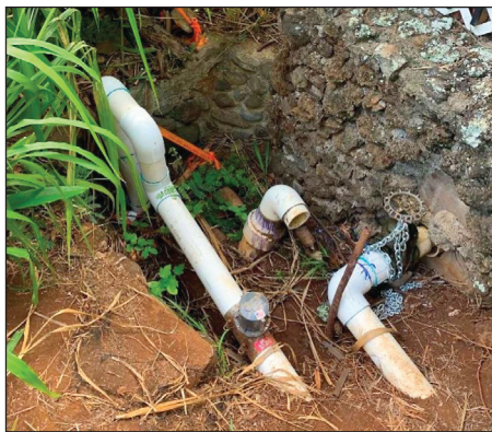
The chained water valve and pipe that releases water into the Wailuku Town kuleana 'auwai.
